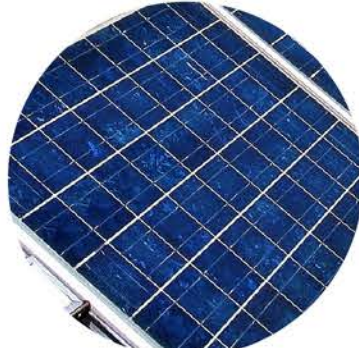
Photovoltaic panels on the roof
